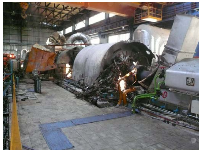
Figure 1: The Iranshahr thermal power plant following a catastrophic wreck of one of its four identical 64MW steam turbine generator trains.
